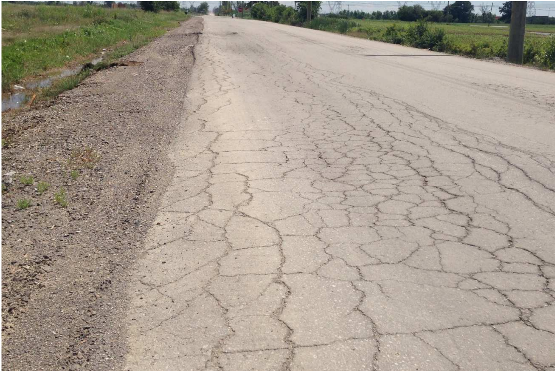
Photo 5: Slight to moderate alligator pavement edge cracking
