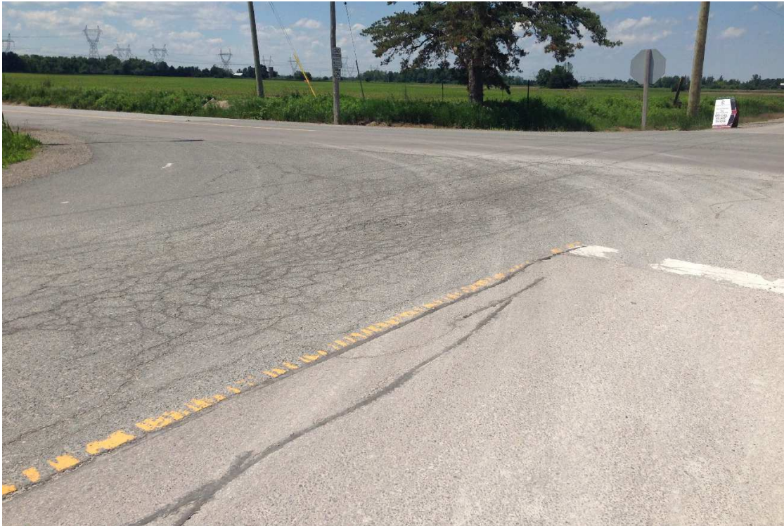
Photo 1: Moderate alligator cracking at south-west corner of Major Mackenzie Dr and Huntington Rd intersection
