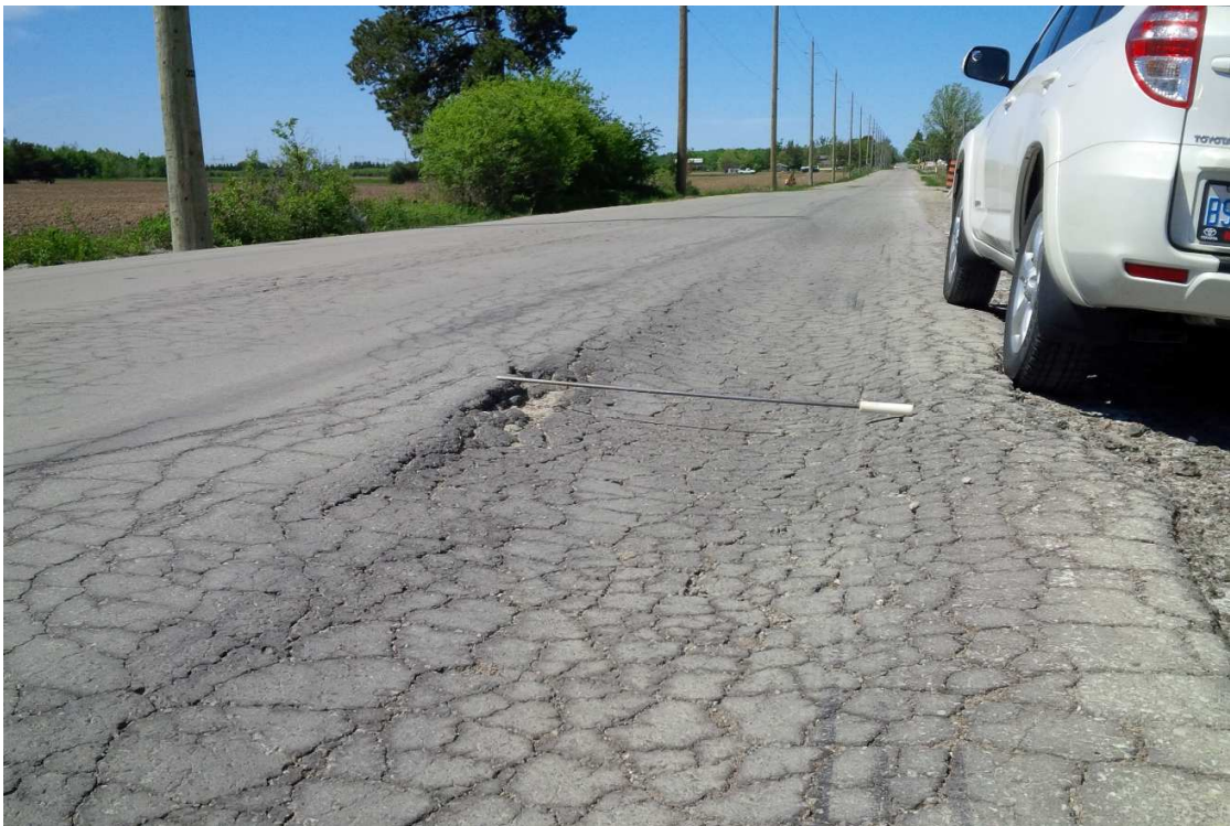
Photo 4: Severe to very severe alligator cracking with potholes from missing blocks
