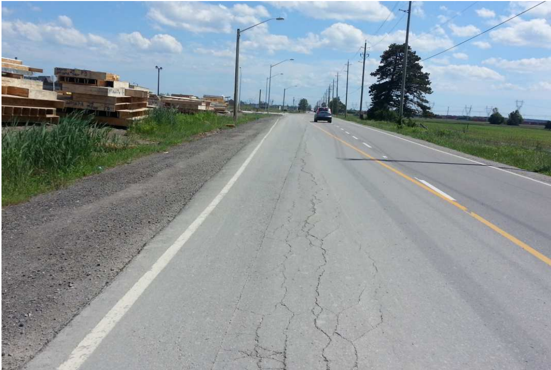
Photo 11: Extension to the road and slight to moderate longitudinal cracking along the construction joint
