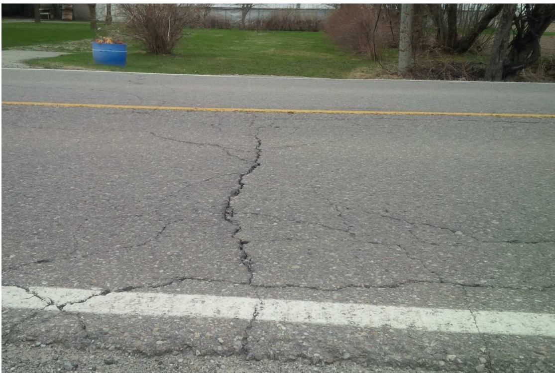
Photo 14: Slight to moderate half transverse cracking and wheel track rutting
