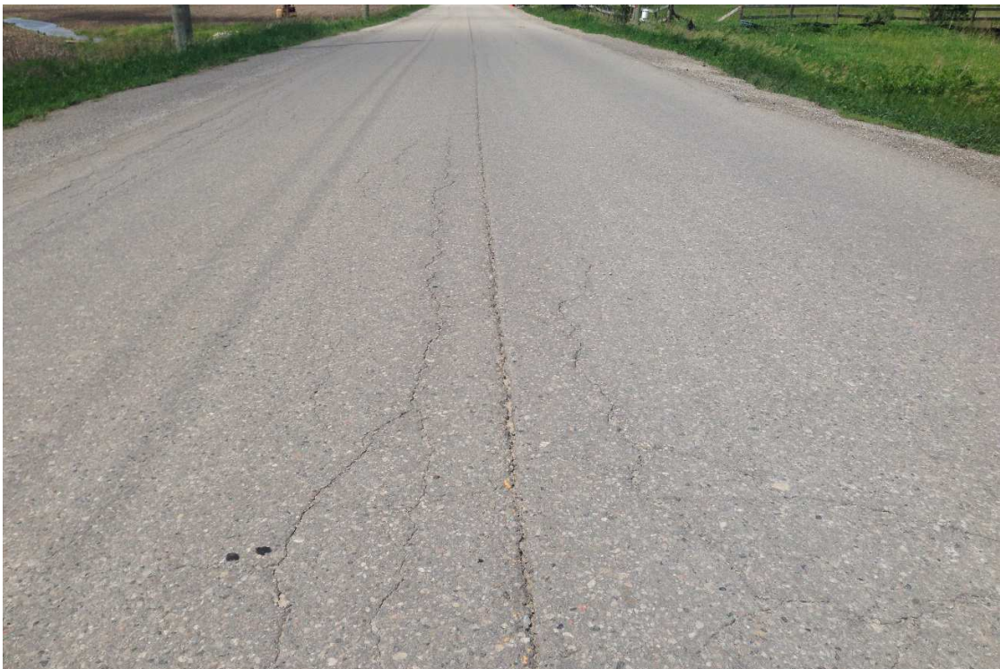
Photo 6: Slight to moderate longitudinal construction joint
