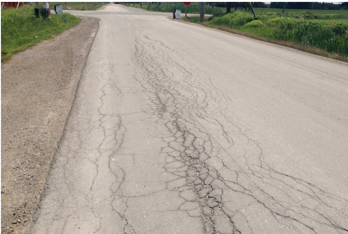
Photo 2: Moderate to severe alligator cracking with small potholes
