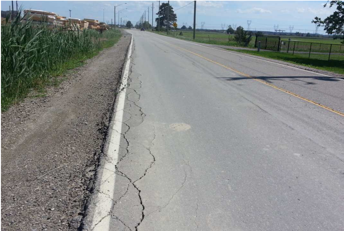
Photo 13: slight to moderate pavement edge cracking along the edge of patched section
