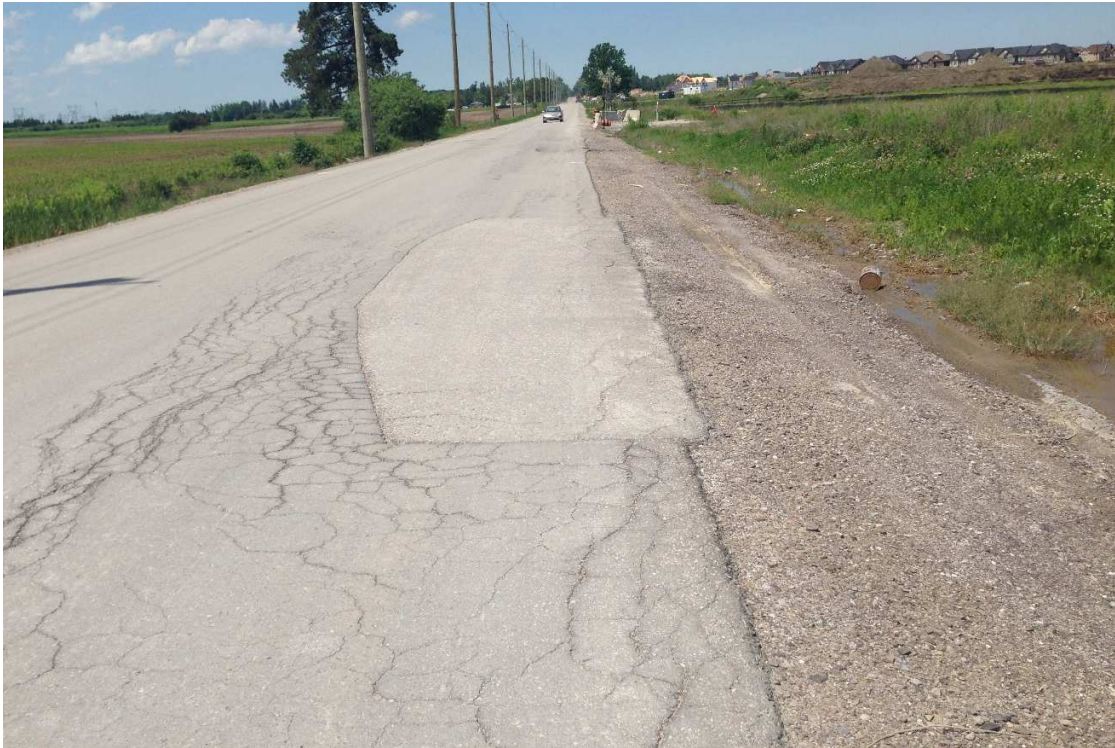
Photo 3: Slight to moderate alligator cracking around patched area and improper ditching along the road
