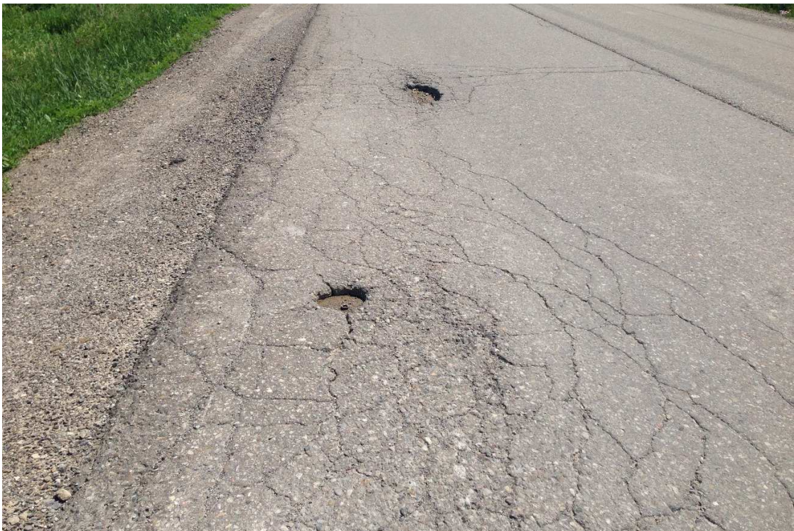
Photo 8: Moderate to severe alligator pavement edge cracking with potholes
