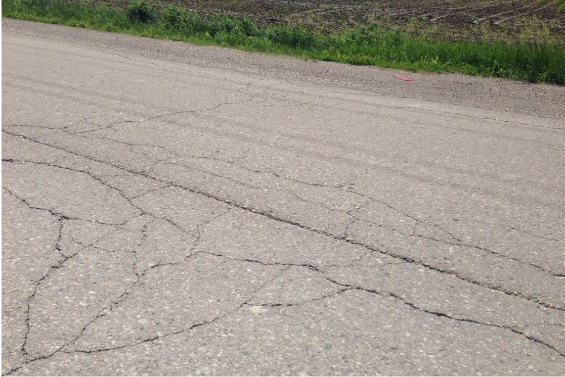
Photo 7: Slight to moderate alligator centerline cracking
