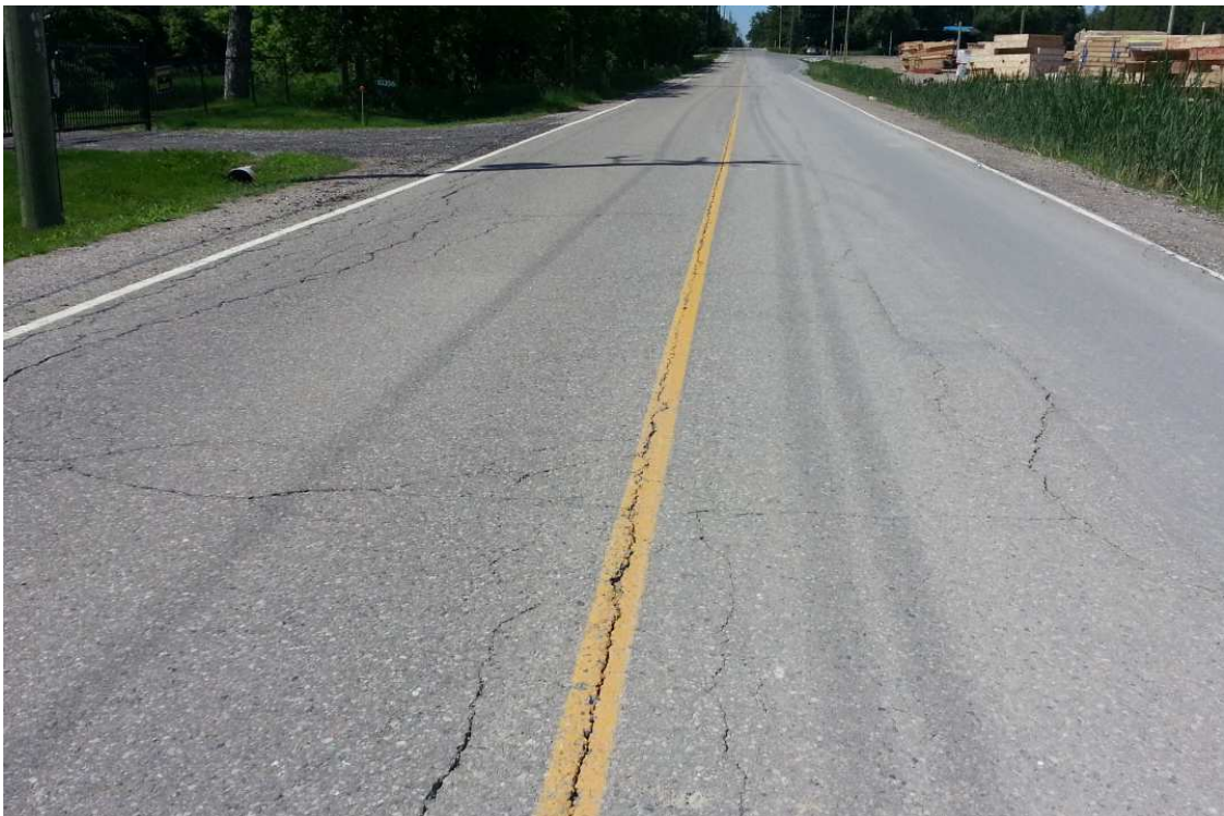
Photo 12: Patching of the road close to construction area, slight to moderate longitudinal construction joint and multiple pavement edge cracking, no proper ditching
