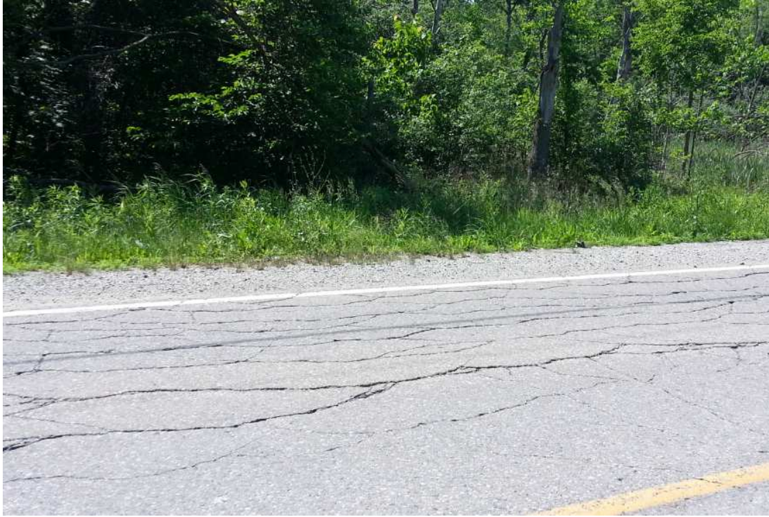
Photo 15: Slight to moderate alligator pavement edge cracking
