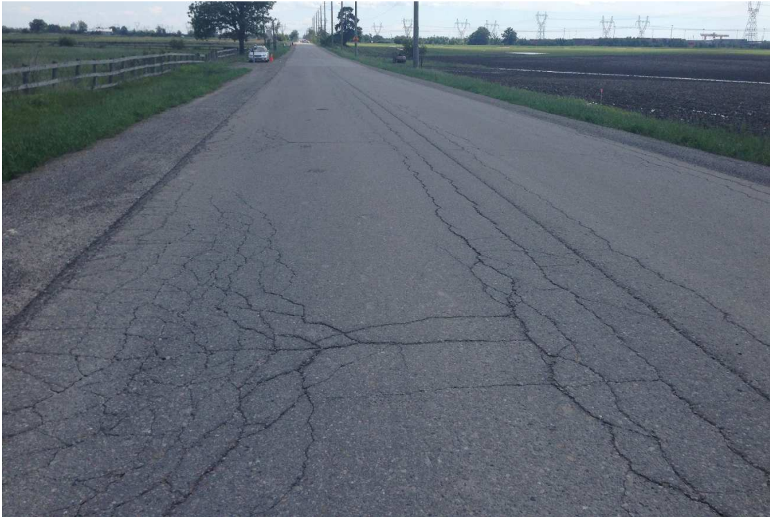
Photo 9: slight to moderate multiple centerline cracking and slight to moderate alligator pavement edge cracking
