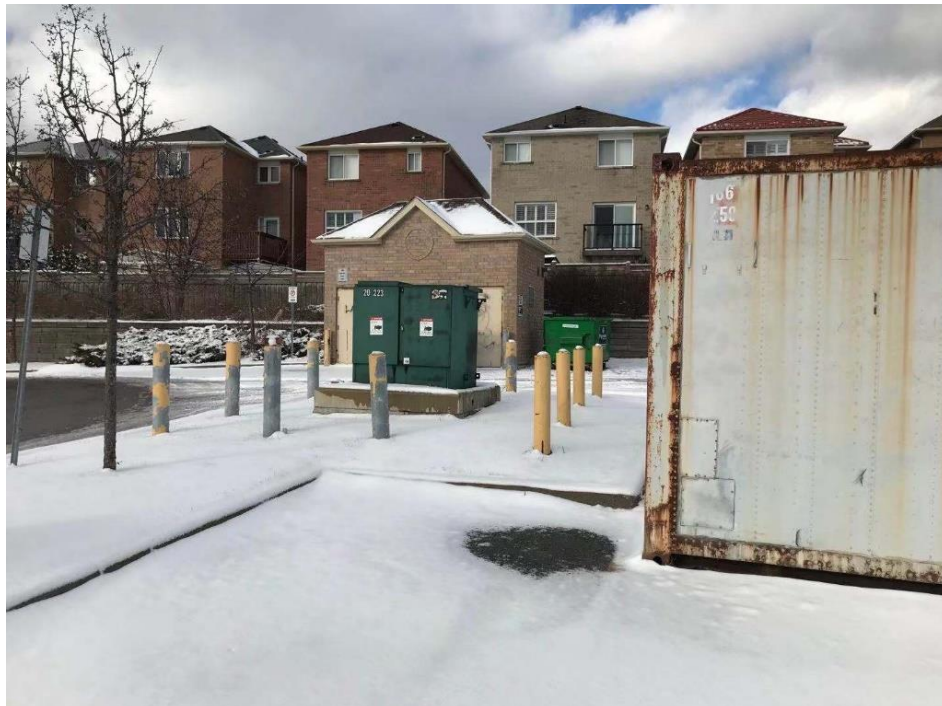
Photo 10: A view of a pad-mounted transformer at the plaza with the municipal address of 11399 Keele Street.
