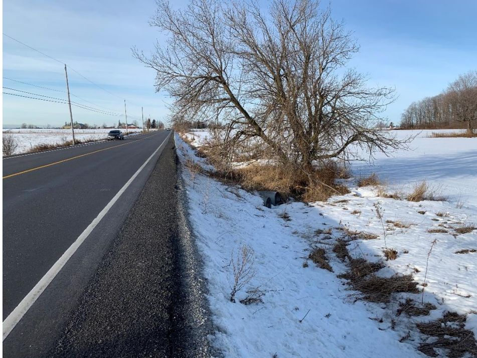
Photo 9: A view to the west on the north side of Kirby Road noting the culvert pipes that extend beneath the Site alignment.
