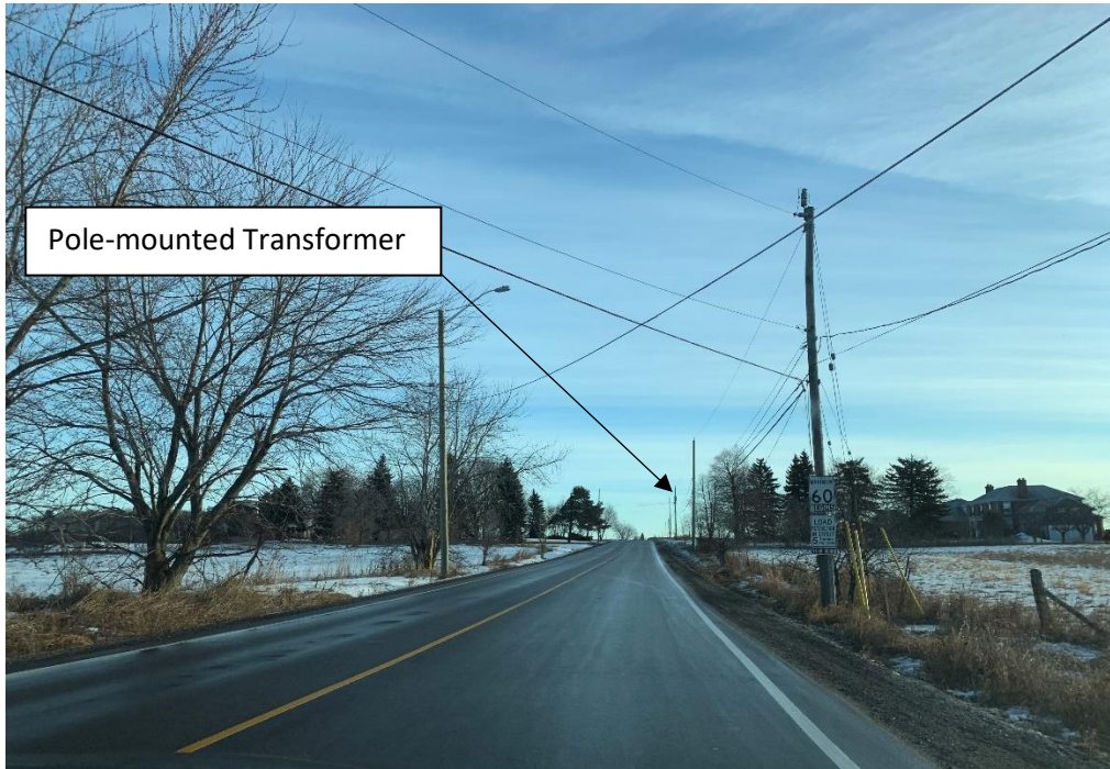
Photo 1: View to the east on Kirby Road from near the intersection of Jane Street. Hydro poles and pole mounted transformers existed on the south side of the road.
