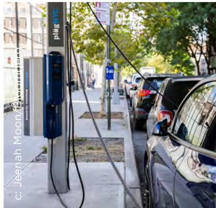
Figure 4.27. EV charging in parking lane.
