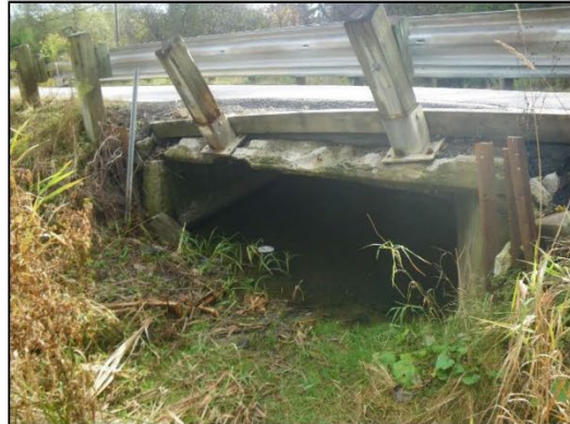
Upstream end of culvert at Crossing C2 facing downstream (southeast). Note pool of standing water inside culvert and dry channel upstream
