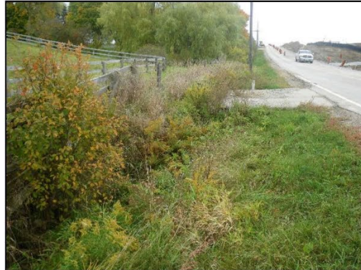
Upstream end of culvert in ditch (adjacent to shrub) with pond in background (behind willow tree). Facing upstream (east) along north ditch of Teston Road
