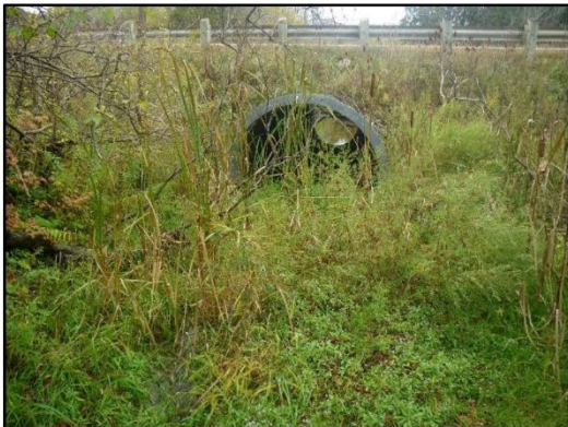
Downstream end of culvert facing upstream (north). Note narrow channel in foreground
