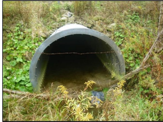
Upstream end of culvert facing downstream (south). Note obstruction from wooden fencing material
