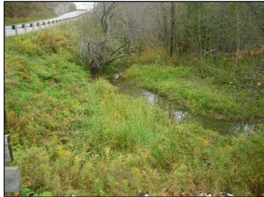
Channel where meander abuts road slope. Facing downstream (east). Teston Road in upper left
