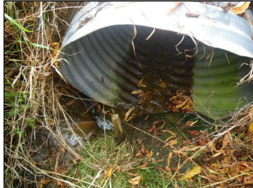
Upstream (north) end of CSPA culvert under Teston Road. Note staked filter sock across inlet
