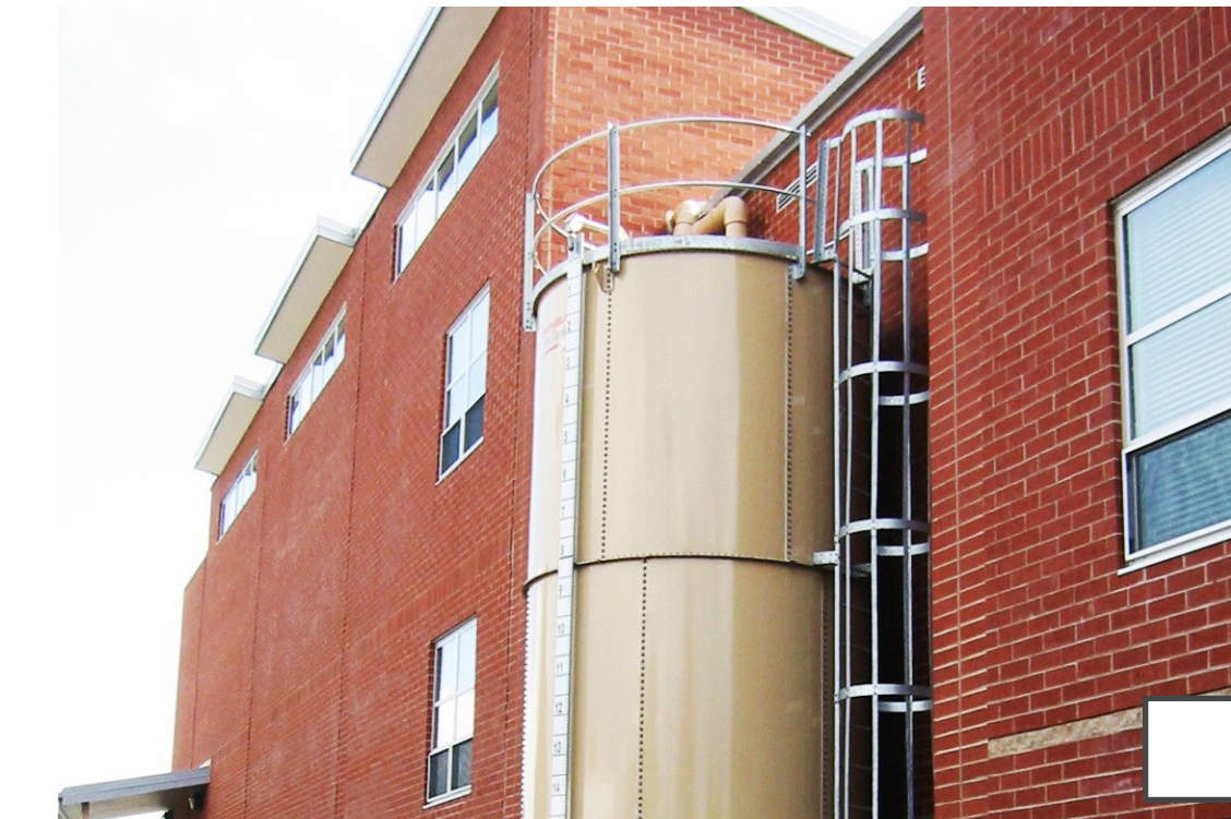
Cisterns and greywater retention for on-site use.
