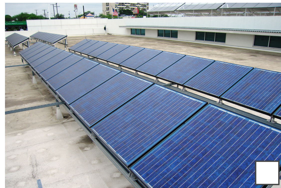
Photo-voltaic and/or Photo-thermal solar energy.
